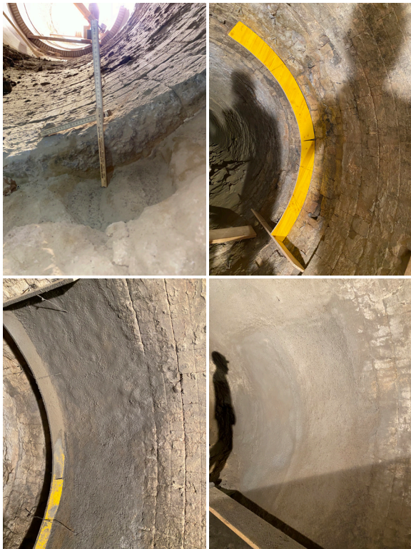
South Austria: Old masonry and discernible thickness of application, field grading, final result after installation.
